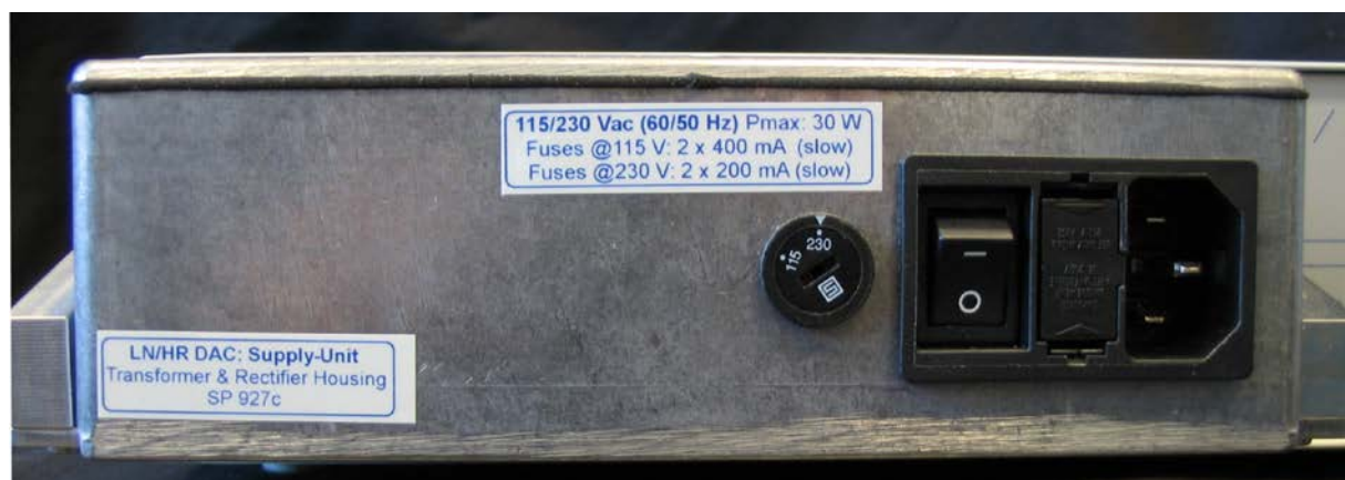
Photo 3: The external and well shielded Transformer & Rectifier Housing on the rear-panel of the LNHR DAC prevents from mains-disturbances.
